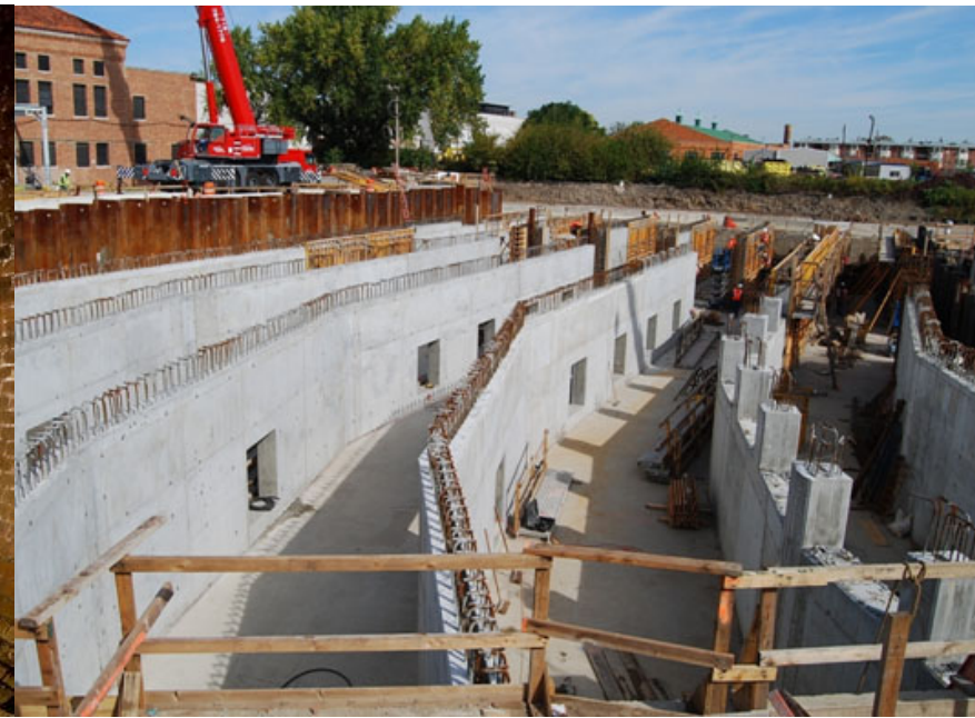
CSO Storage Facility-Brooklyn
