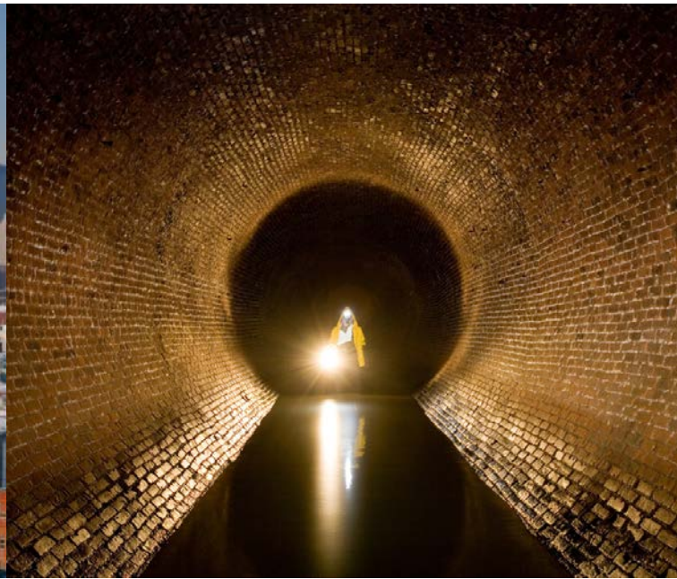
Combined Sewer Pipe-Brooklyn
